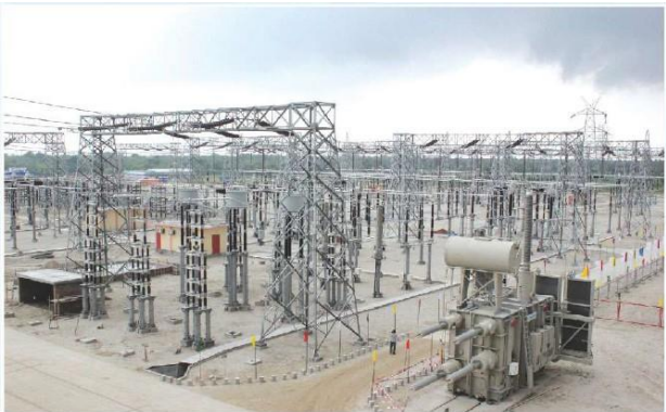
Figure 17: Bangladesh India Power Transmission Plant, Bheramara (Kustia)
