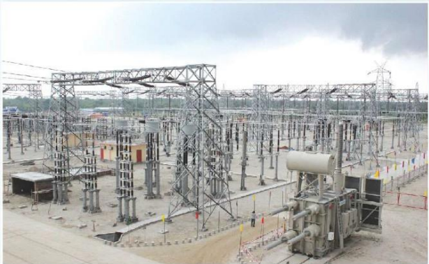
Figure 17: Bangladesh India Power Transmission Plant, Bheramara (Kustia)
